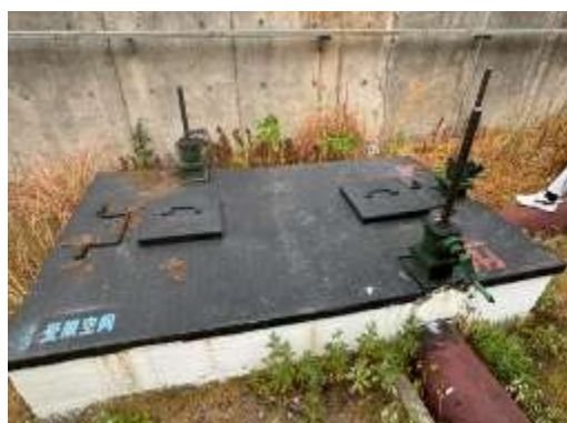
罐区水封井、雨污水切换阀
